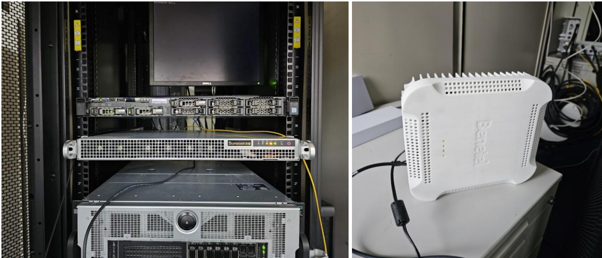
Figure 5-11 Physical installation of ACC O-RAN BS @ OTE testbed
